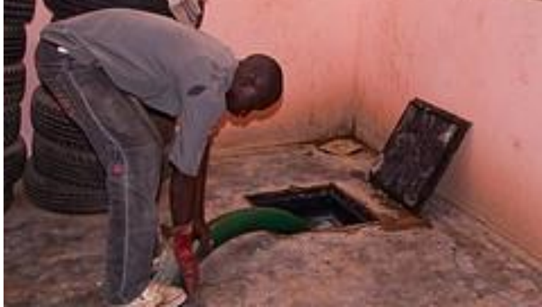
Septic tank (Dakar, Senegal)
